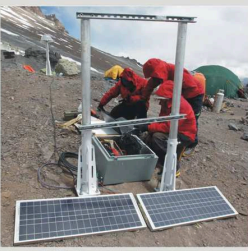
Solar panels structure
